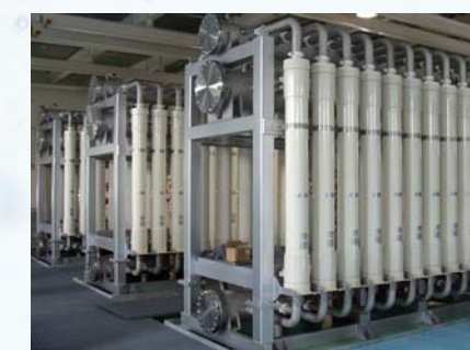
Drinking Water Production Capacity: 44,000m 3 /d x 2 plants Location: Tokyo, Japan Operation start: Mar. 2007
